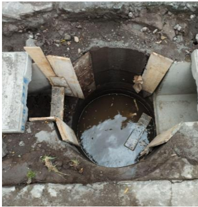
(a) Infiltration Well in Neighborhood Road
