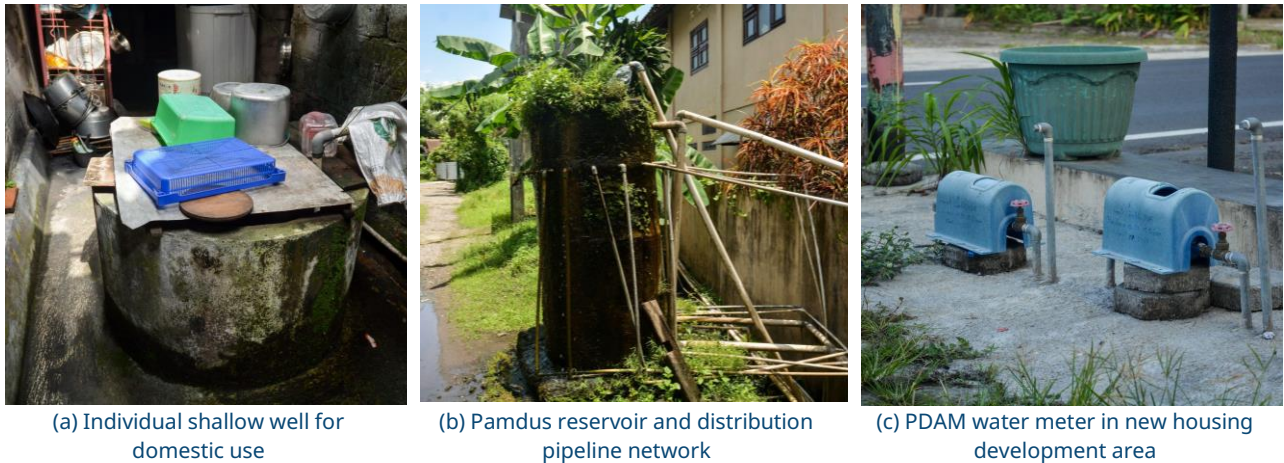
Figure 3.20. Water supply resources in Rejodani Source: Field Observation, 2024
