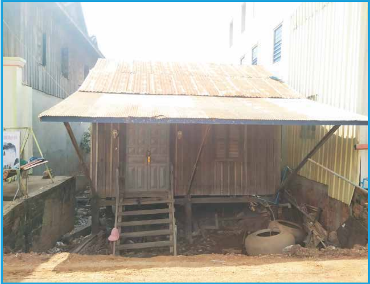
Figure 53 Potential accumulation of rainwater due to adjacent construction walls on property boundaries (Source: Own Photo taken in 2019)
