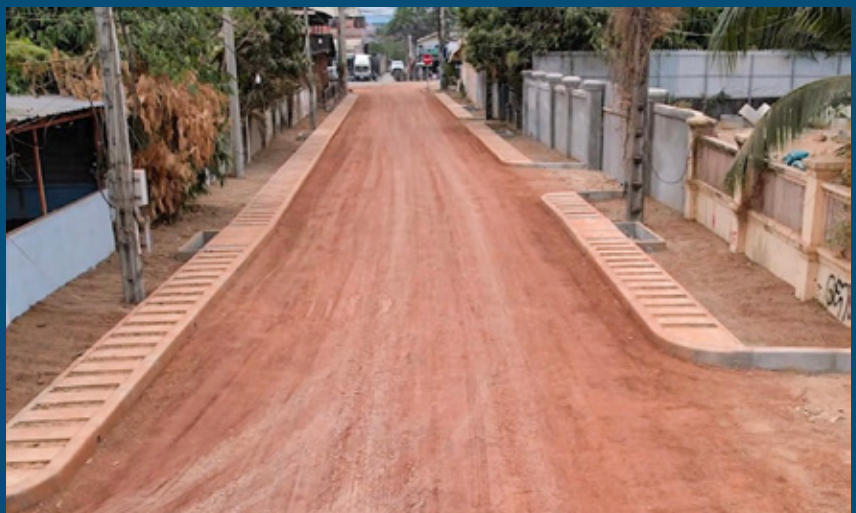
Final improved drainage system (Source: BORDA-Cambodia)
